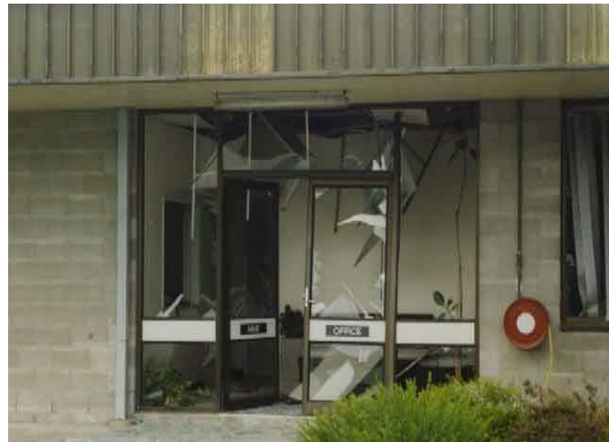
Offices at Huntly West Mine after the explosion. (2005.196.17)
